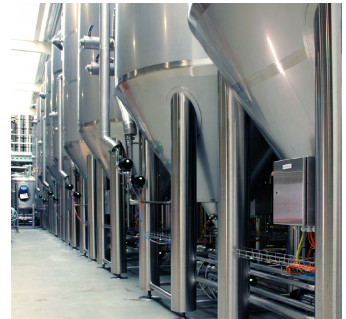
GEA fermentation tanks
